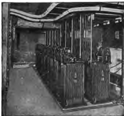
FIG. 174. Installation of General Electric automatic induction feeder regulators at the Philadelphia Electric Co.
